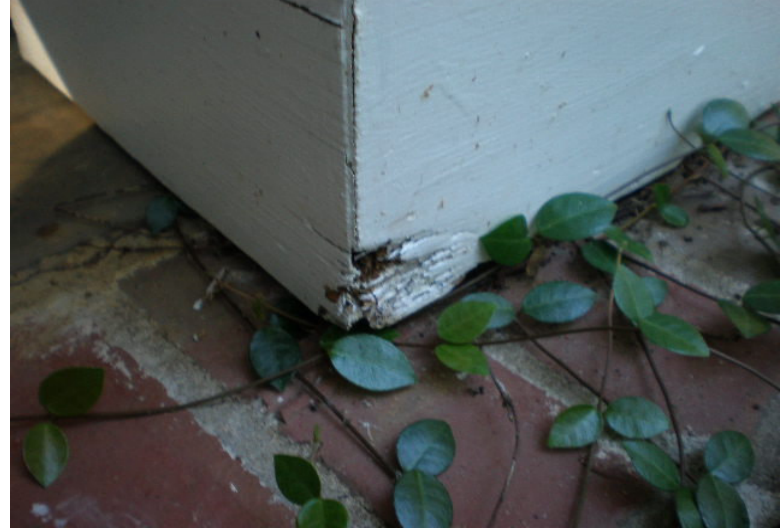
213. Exterior Wood Rot/Decay
