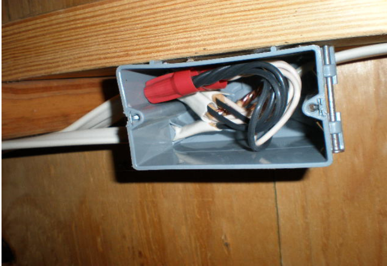
533. Open Junction Box/No Cover
