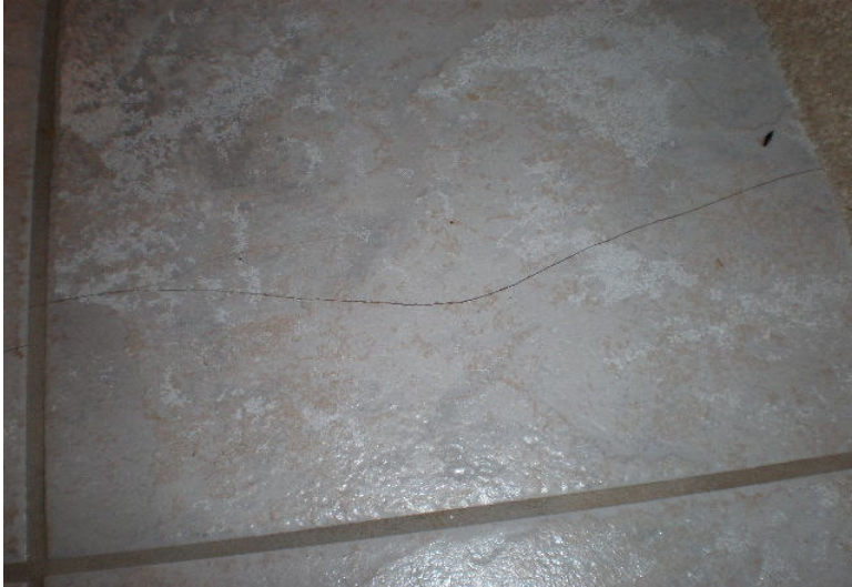
807. Cracked Floor Tiles
